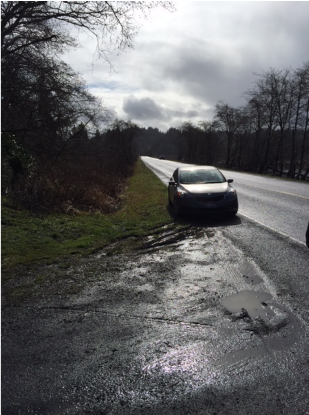
Photo 5. View southeast along N. Beaver Creek Road. Raw water pipeline to be located in the southwest lane (right side of this photo).
