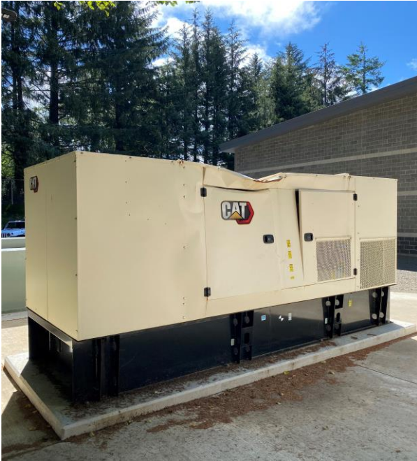
Damaged Standby Generator Housing:
