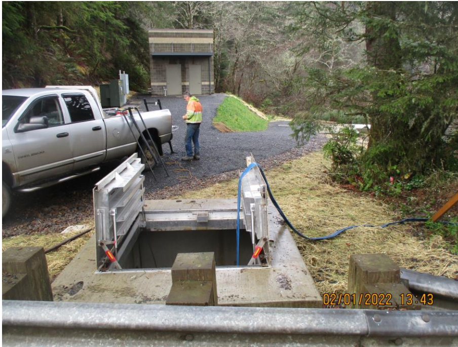
Beaver Creek Intake and Valve Vault:
