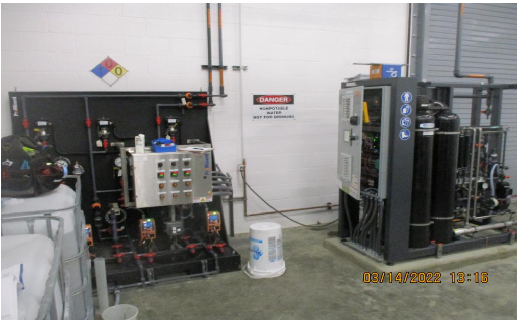
Onsite Chlorine Generation System:
