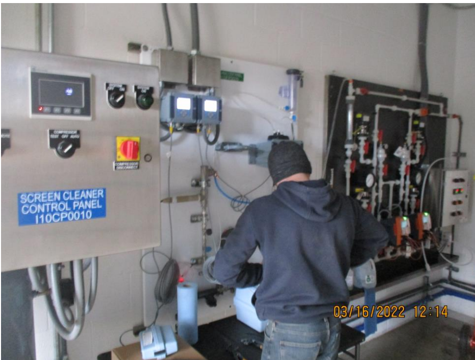
One of the many Control Panels:
