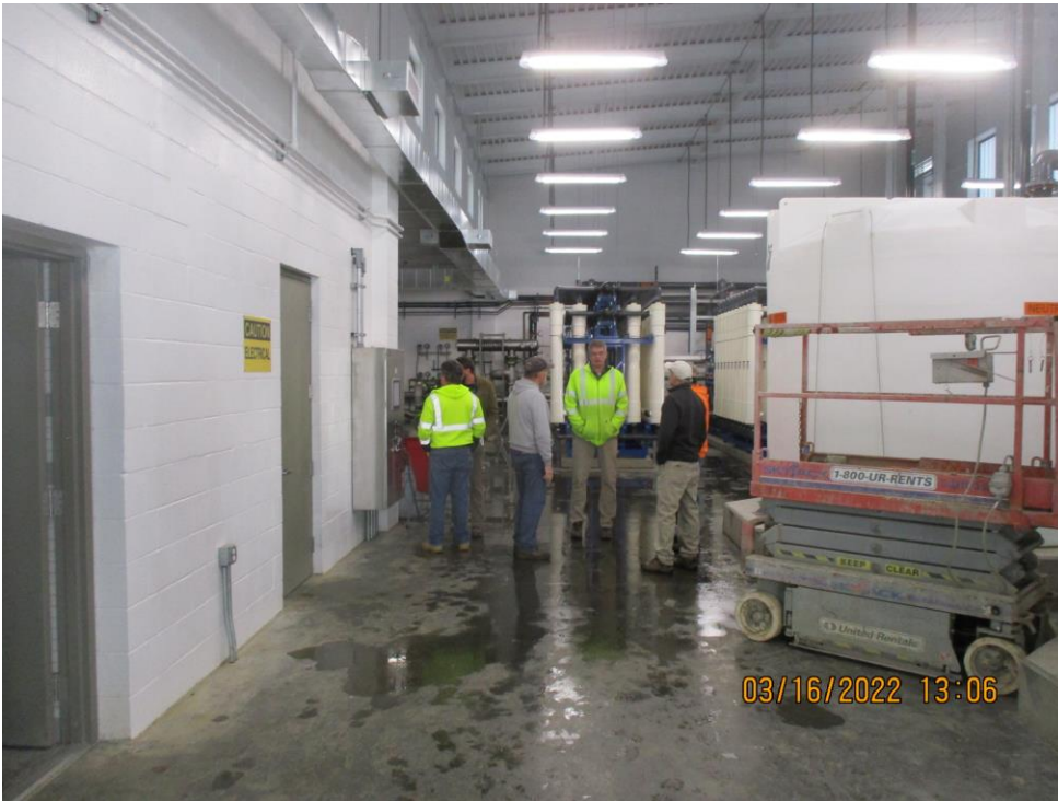
Water Treatment Plant Membrane Banks in the Background:
