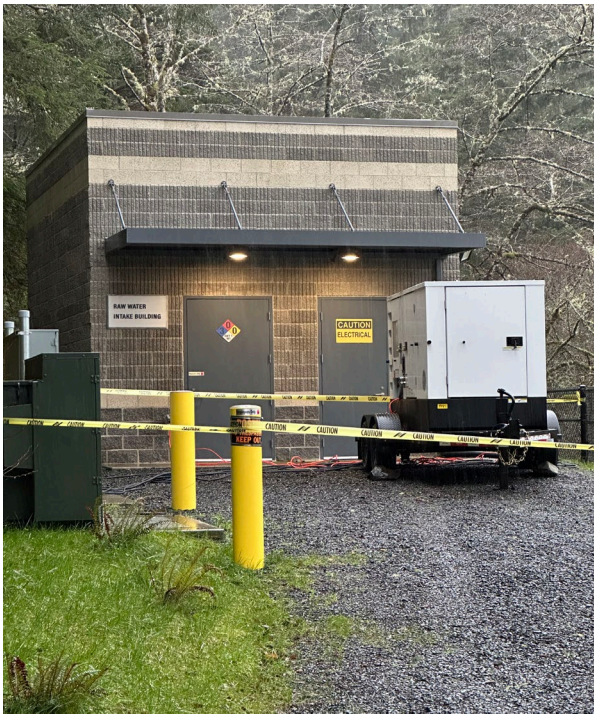
Portable Generator at the Beaver Creek Pump Station:
