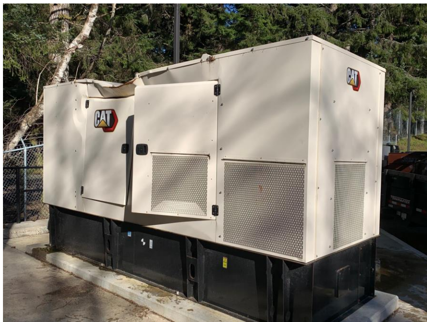
Damaged Generator Housing:
