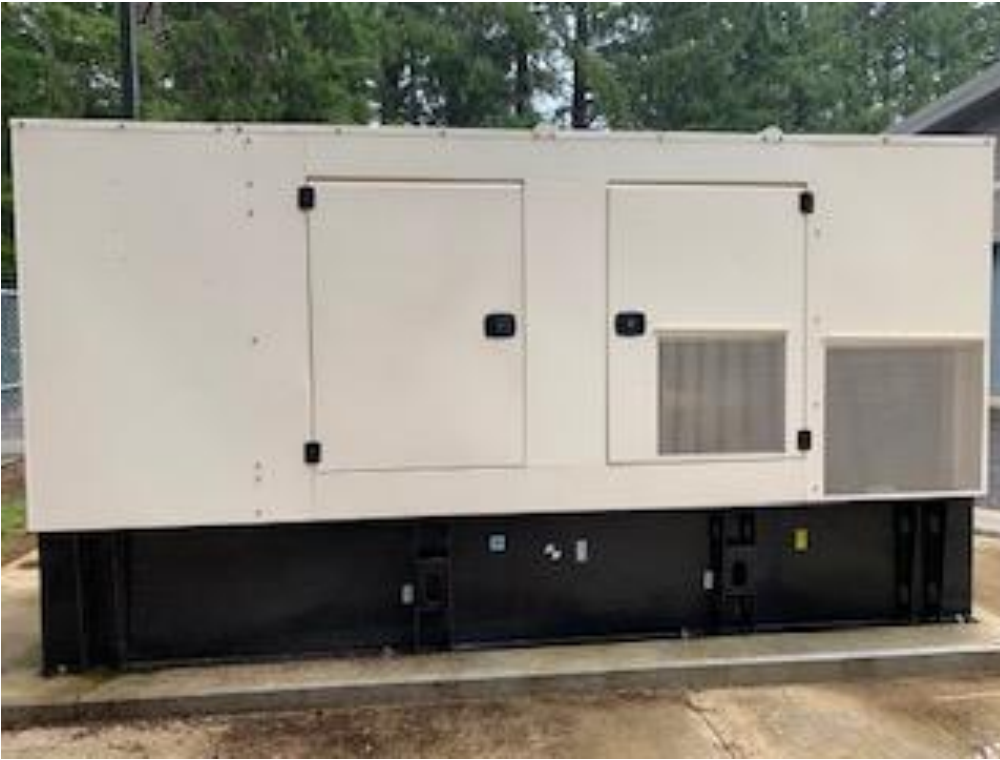
Newly Installed Generator Housing:
