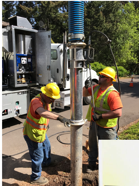
SRWD Distribution Operators safely maintain over 65-miles of distribution system.
