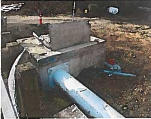
Piping south vault:
