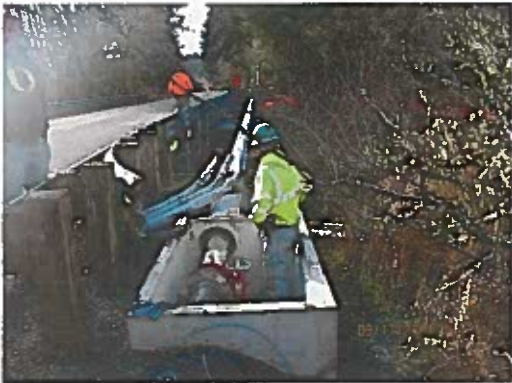
Bridge piping north vault:
