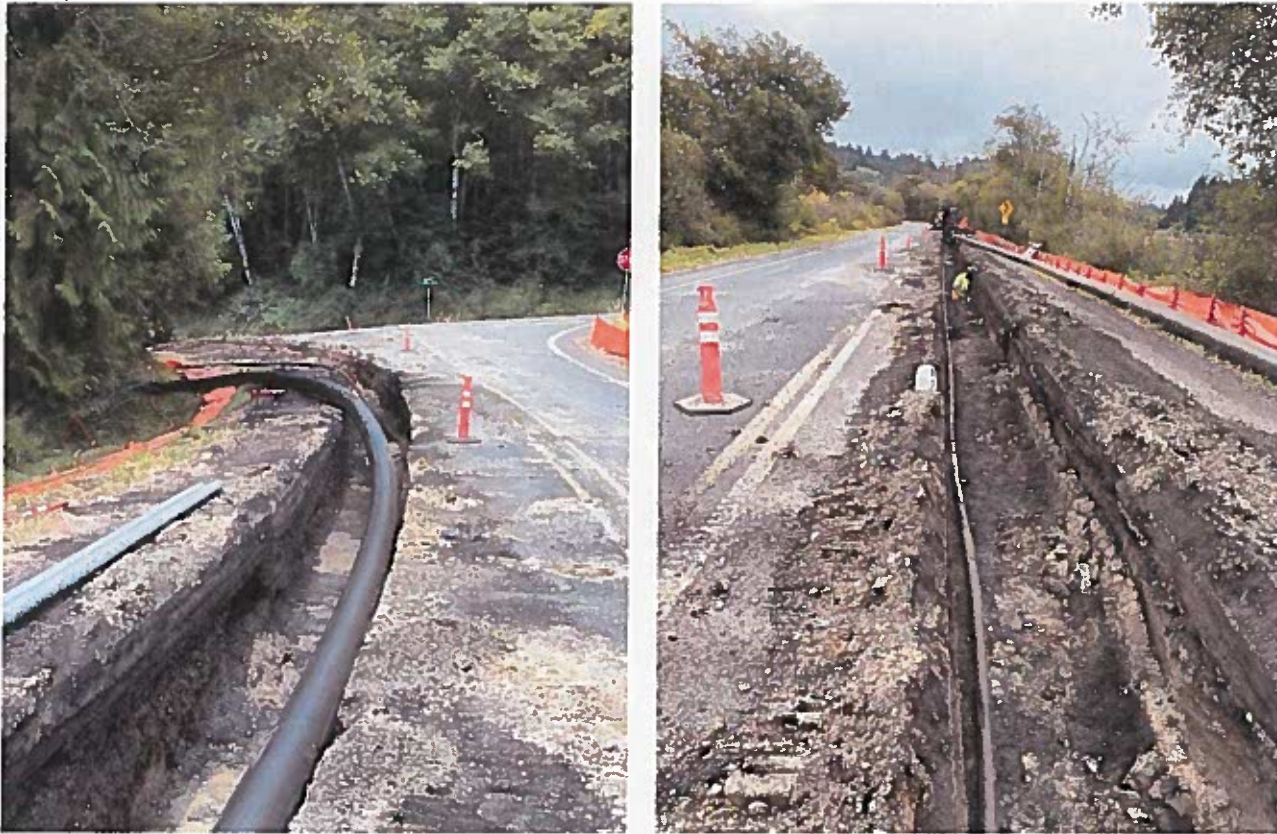
Beaver Creek Source Water Project, Raw Water pipeline installation along Beaver Creek Road:
