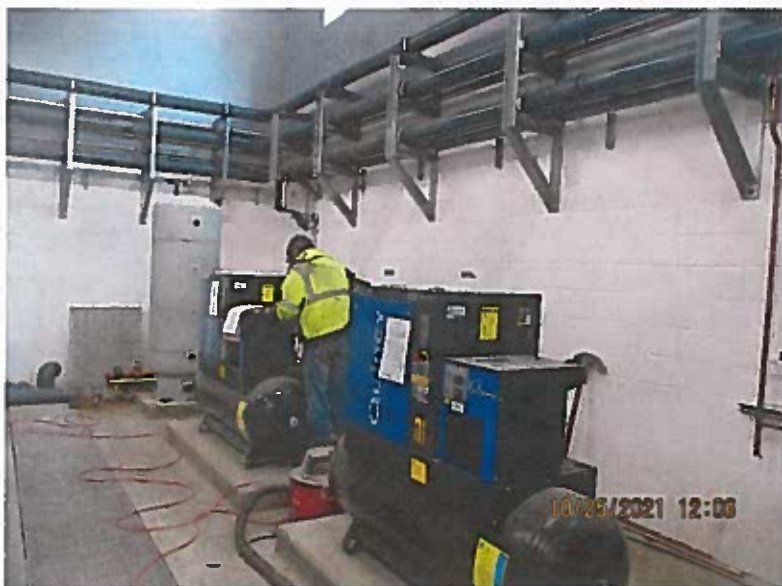
Air Compressors/Treatment Building:
