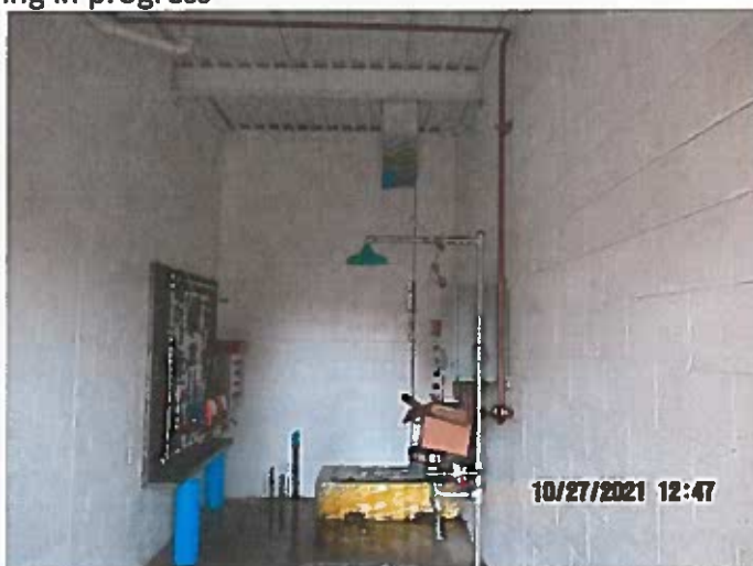
Beaver Creek Intake, Pre-Treatment Room:
