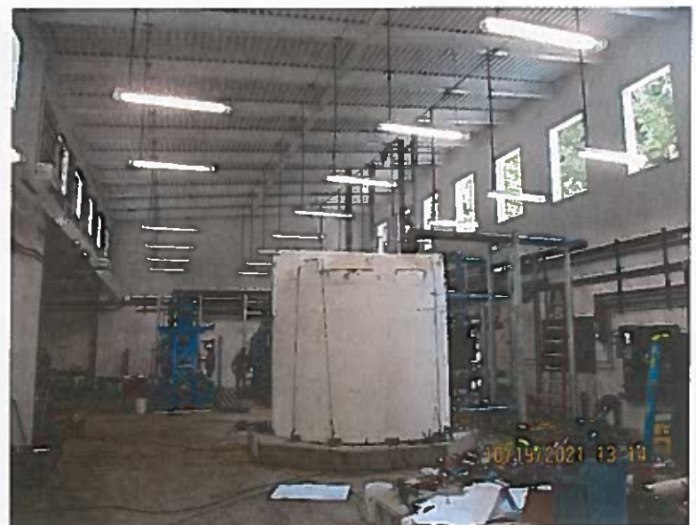
Solution Tanks/Treatment Building:
