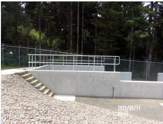
Safety Railing Around Backwash Basin:
