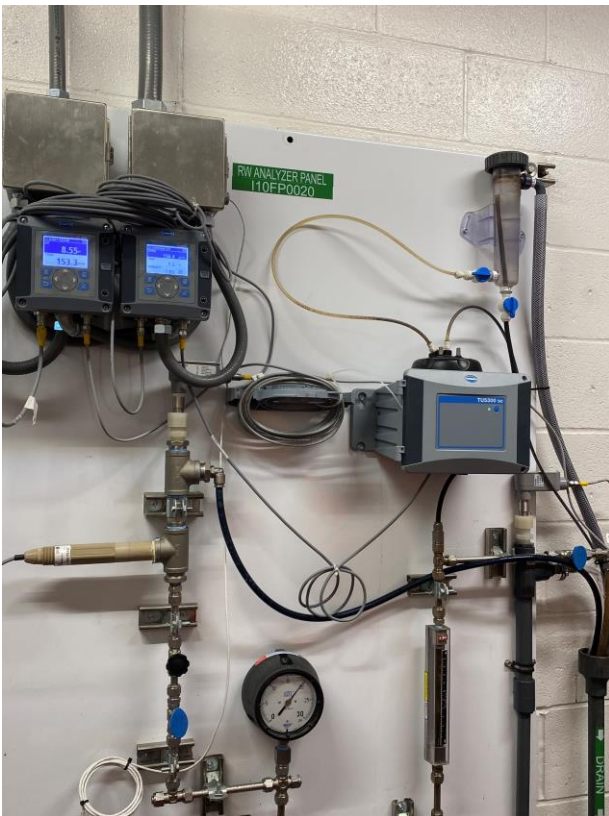
Above: Raw Water Intake Redundant Conductivity Probes and readout panels
