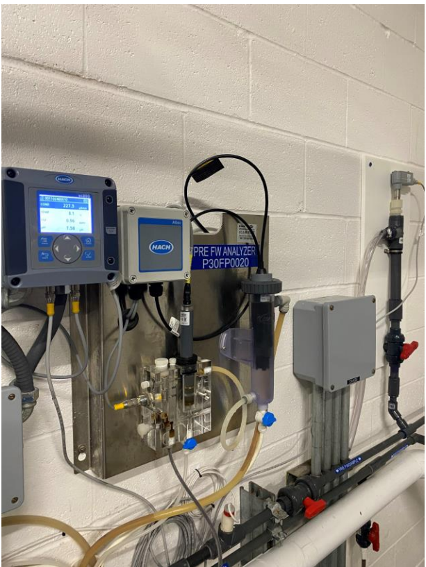
Above: Finish Water Conductivity Probe with readout monitor at the Water Treatment Plant
