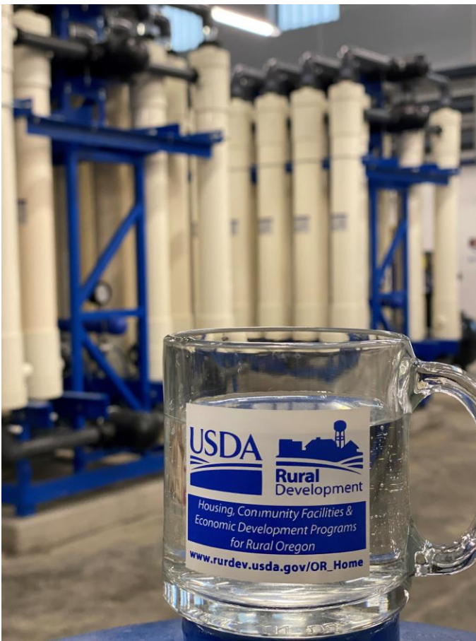
Membrane Filter Racks:
