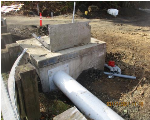
Piping south vault:
