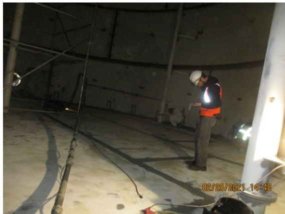
Interior of clearwell:
