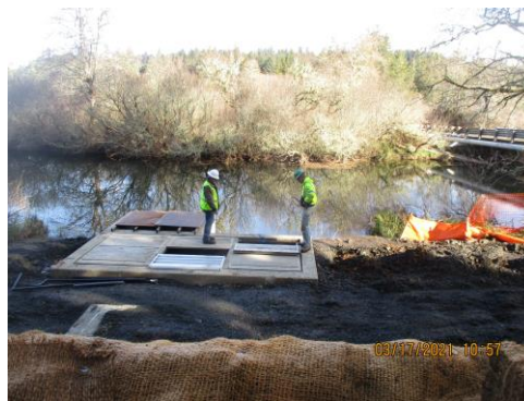
Intake with hatch covers:
