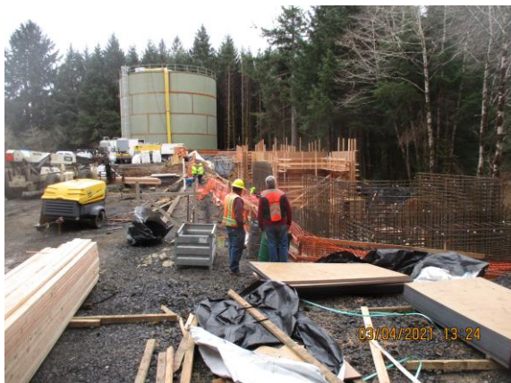
Clearwell and Backwash Basin:
