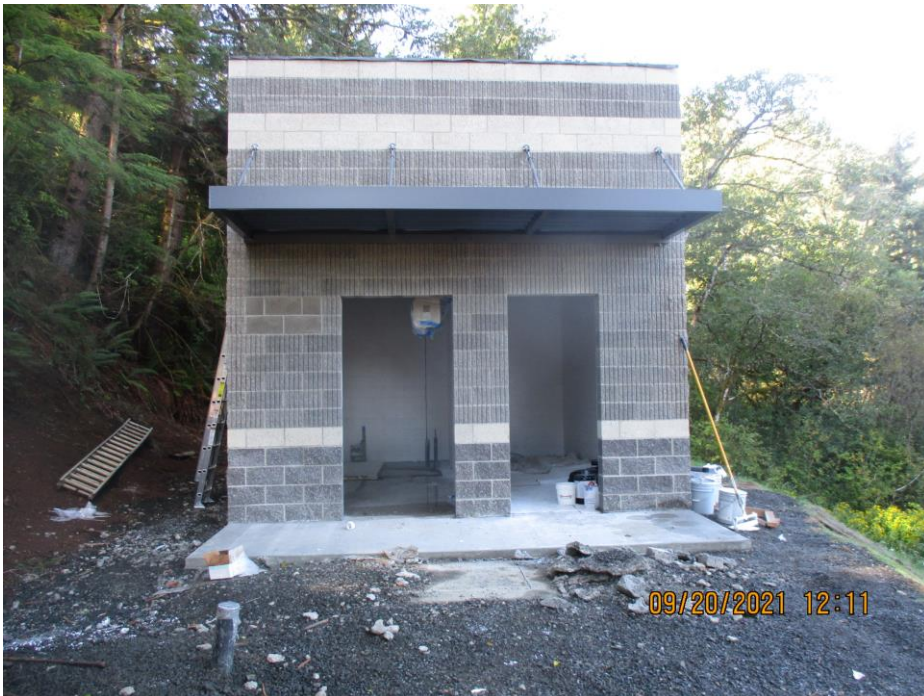
Intake Electrical Building:
