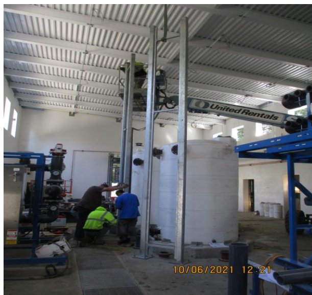
WTP Mixing Tanks:
