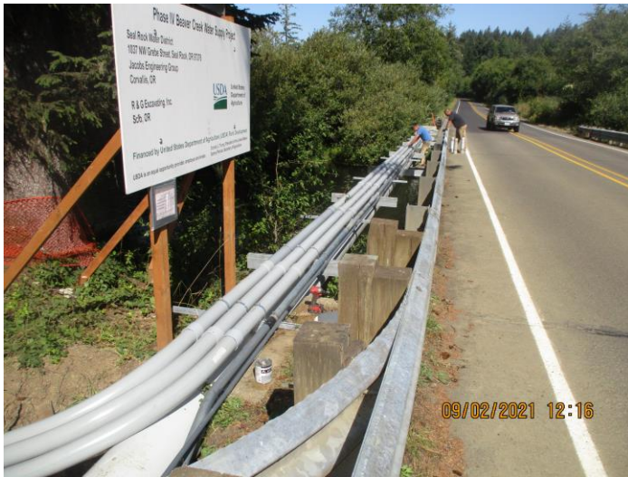
Pipe gallery across Beaver Creek Bridge:
