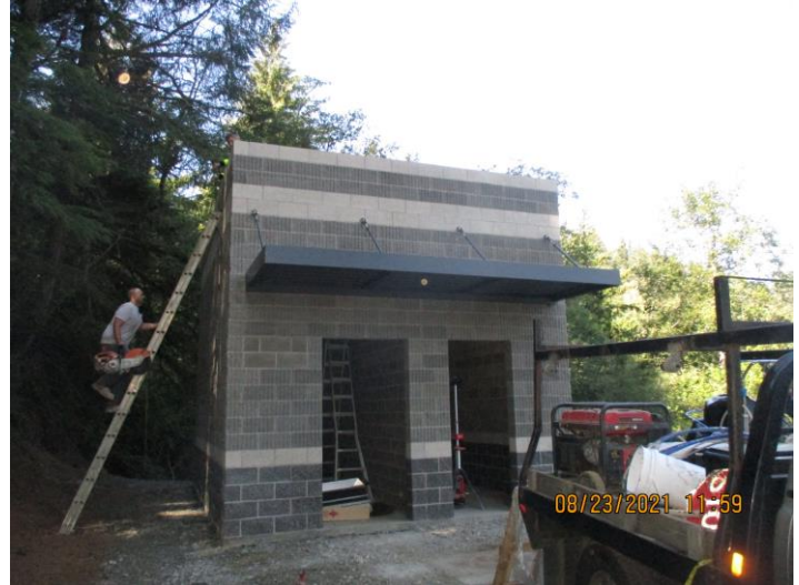
Intake Electrical Building:
