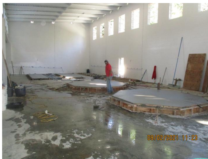
Interior Membrane Building:
